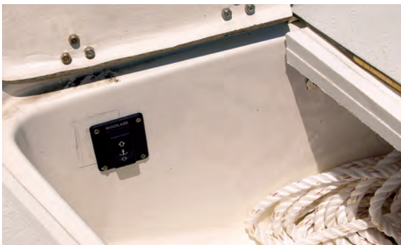
Clarence put the windlass master switch in the anchor locker, above. Note the hatch latches, at right.
