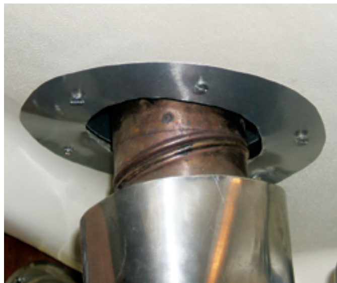
Metal trim rings shield the deck from the hot flue.
