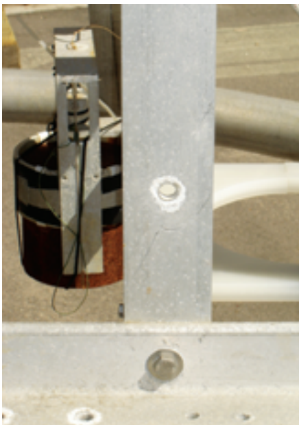
Aluminum corrodes when it's in direct contact with stainless-steel fasteners.
