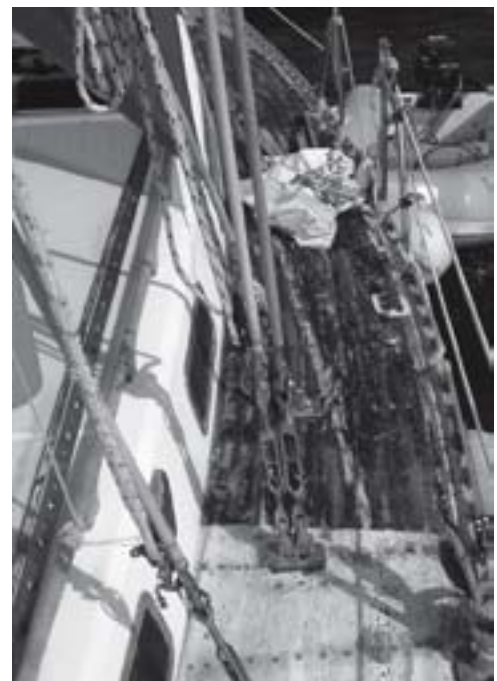
Doug removes the last piece of teak, at top. The tar bedding, at right, was removed with diesel fuel.
