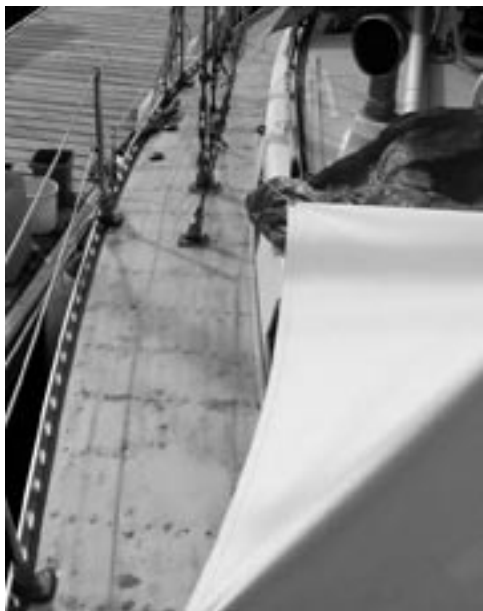
With the teak and the goo gone, Doug con-templates filling all the holes, at top. The prepared deck awaiting the primer coat, above.
