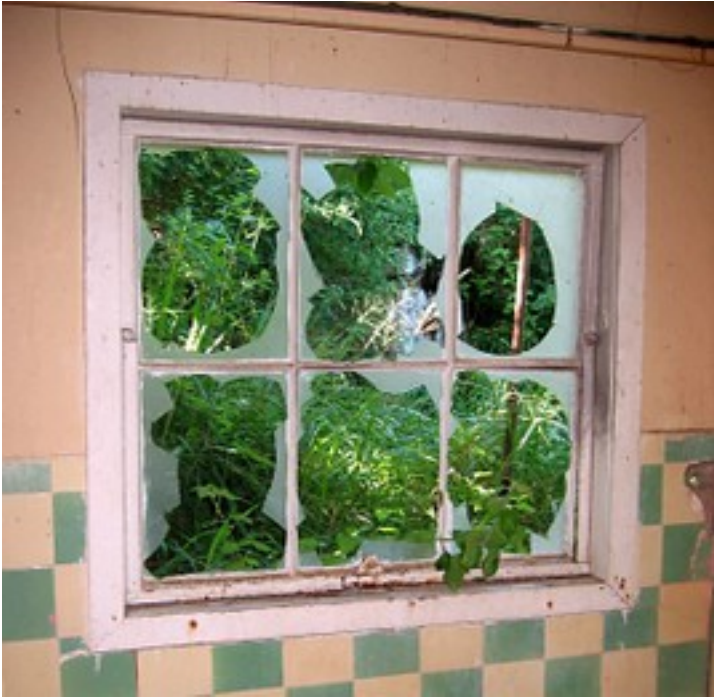
Vandals haven't been kind to the old buildings
