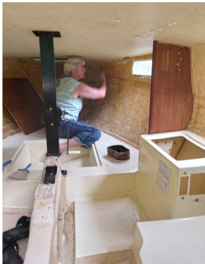
After the old fabric was removed, the walls were scrubbed with 60 grit sandpaper, then painted with mold killing primer.
