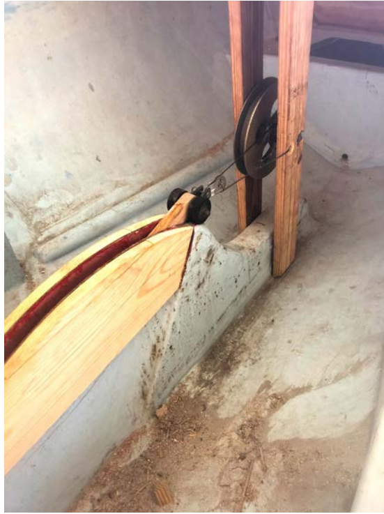
Far left and left, the centerboard trunk was rebuilt to the original design.
