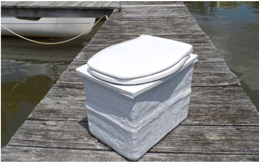
At left and below, Drew used a pair of battery boxes to make the lower part. The unit would be enclosed in a well, but he wanted the toilet to have a smooth, well-finished interior.
