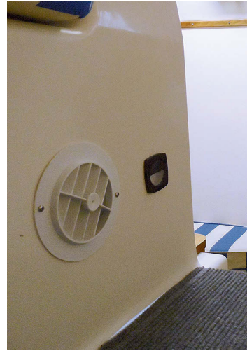
Drew's AC unit was a tight fit under the saloon seat, far left, but there is room to pull it out through the next seat. He mounted this rotatable outlet where it can direct air into the starboard hull or into the saloon, at left.
