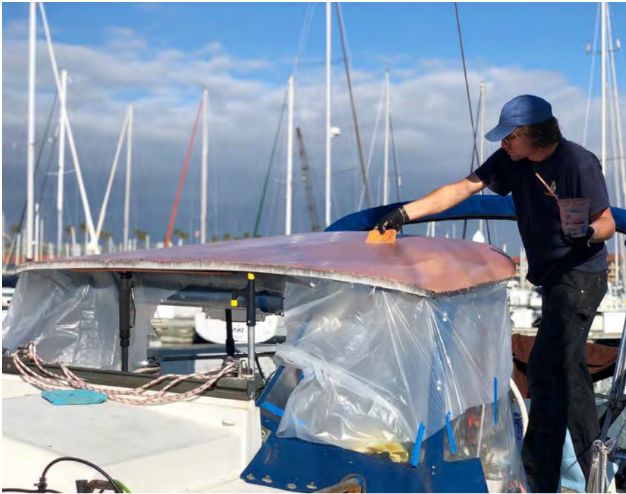
Applying fairing compound to the new hardtop, top left. Note the supports beneath, which Chris added when the new core material developed some dips as glass and fairing were added.
