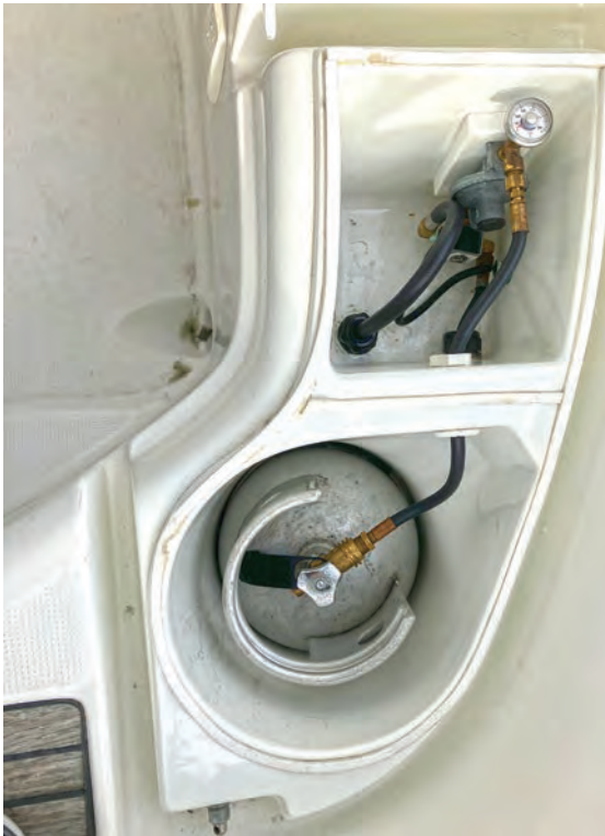
At left, Honcho's dual compartment propane locker.
