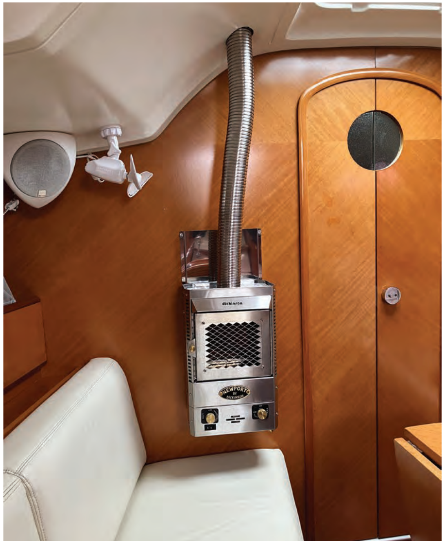
The new propane fireplace connected to the chimney and secured to the bulkhead.
