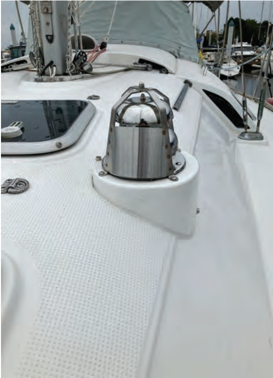
At left, the flue cap and base attached to Honcho's cabin top.
